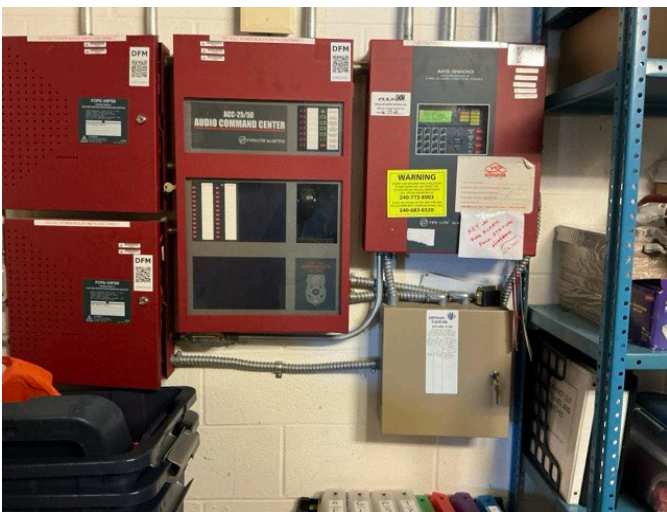
23 - FIRE ALARM PANEL
