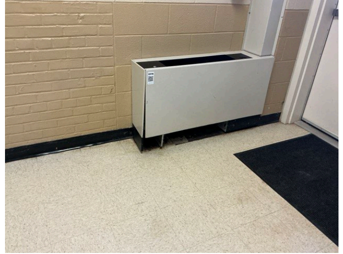
20 - SUPPLEMENTAL HVAC EQUIPMENT
